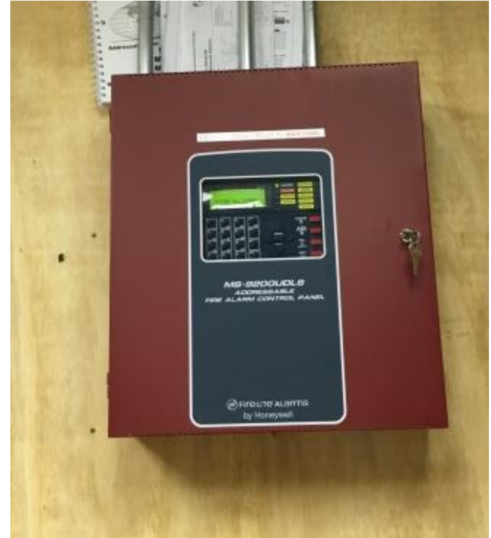
Fire Alarm Panel
